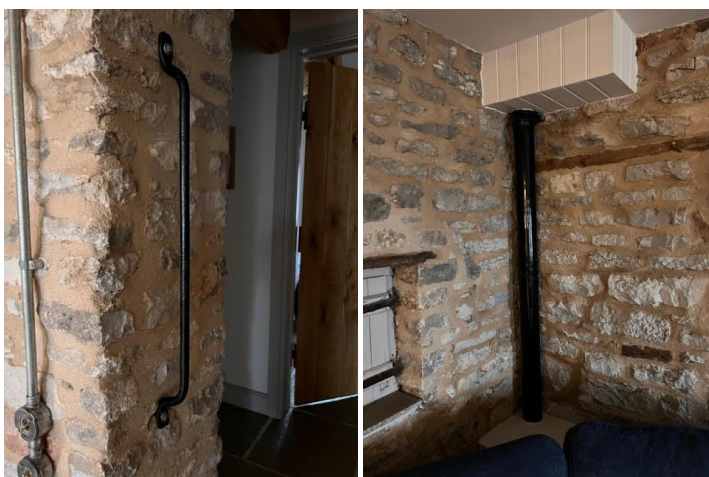
Cattle restraint re-used as hand rail, reclaimed external pipe used as exposed soil pipe, retained feeding hatch, and repointed interior walls.
